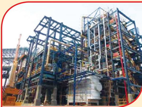
PA Plant Revamp : Oxidation Section - Ranipet
