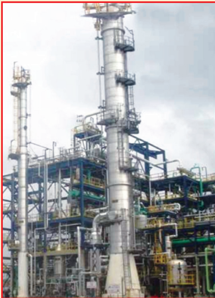
Butane Processing and Butamer Plant: Malaysia
