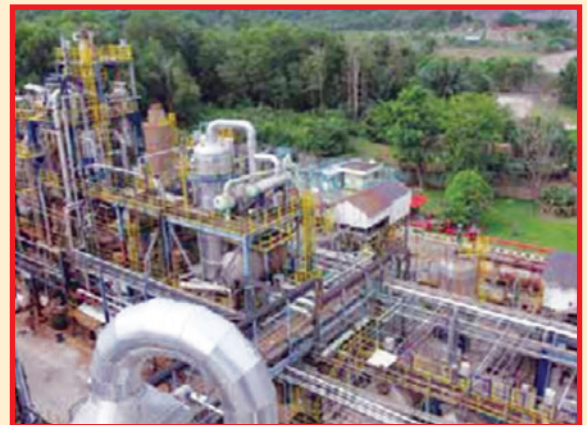
Maleic - Distillation Unit after Expansion : Malaysia
